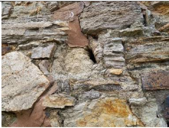
Photograph 9: Gaps in stone on B2
