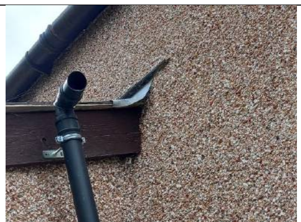
Photograph 6: Lifts in flashing on B1
