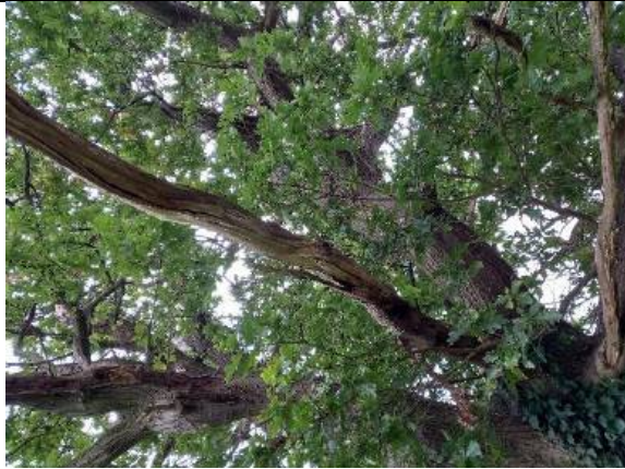
Photograph 19: Broken and split branches of tree T7 (oak) assessed to provide moderate BRP
