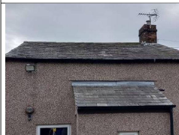
Photograph 5: Lifts in tiles on B1
