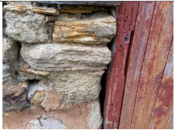
Photograph 10: Gaps between door frames and stonework on B2
