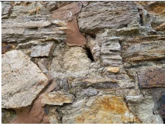
Photograph 9: Gaps in stone on B2
