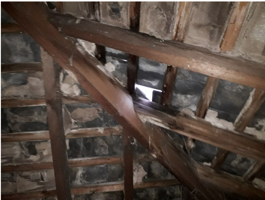
Plate 8. Missing slate within the roof of void 3.
