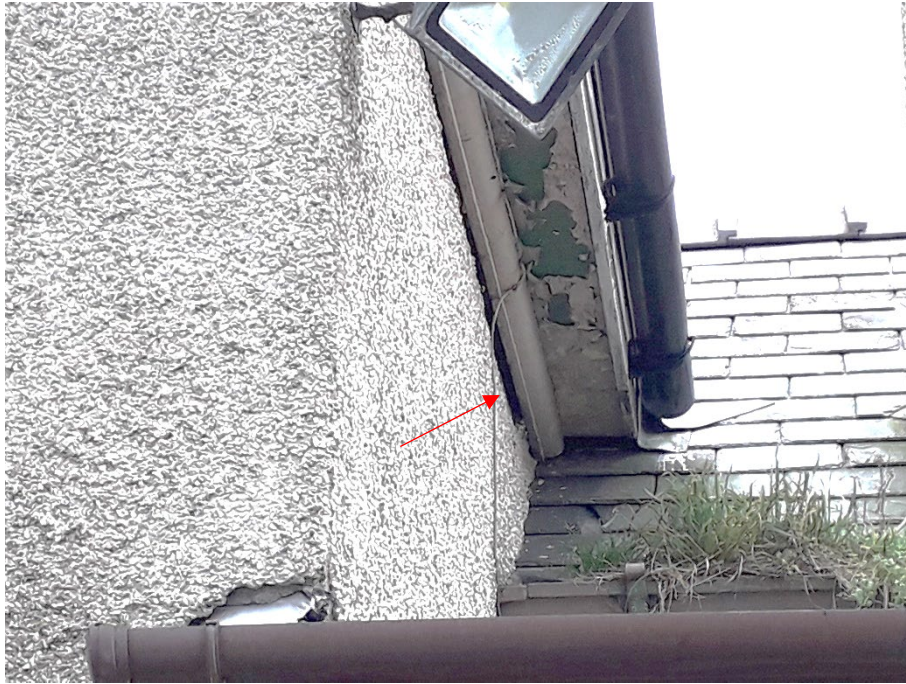
Plate 3. Example of PRF A2 – gap between wall and soffit.
