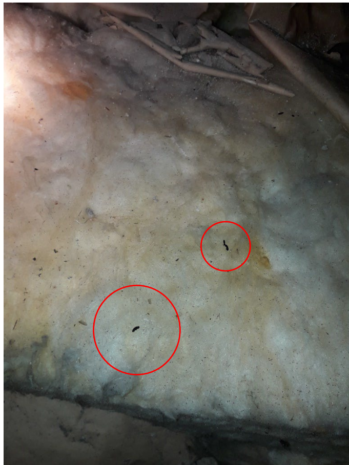
Plate 20. Potential bat droppings in void 2 by the access door to 3.
