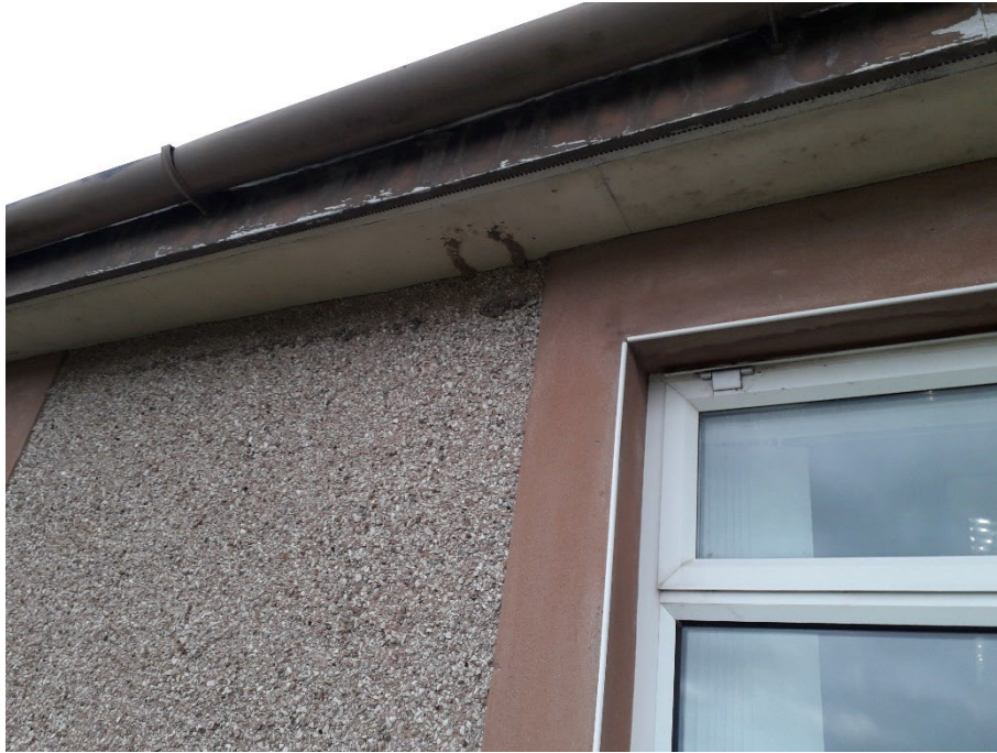
Plate 5. Evidence of potential swallow birds' nest under the soffit.
