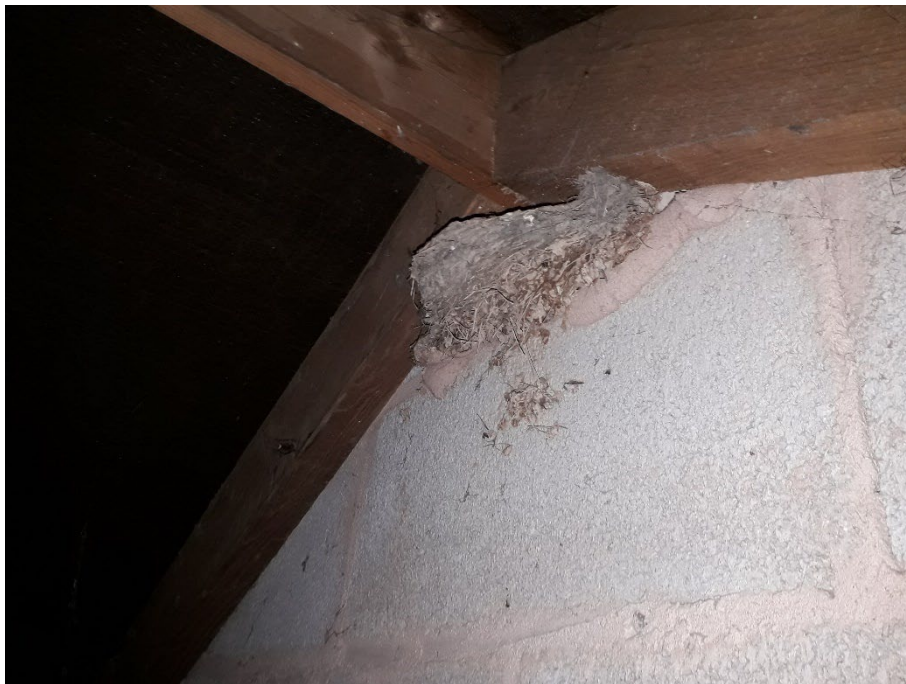
Plate 24. Old birds' nest within one of the central roof voids.
