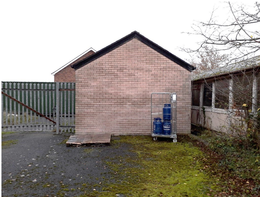
Plate 21. Southern gable end of the building. PRF D1 – gap under the fascia boards.
