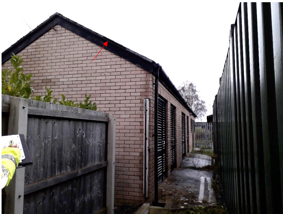
Plate 22. Northern gable end and access door on the western side. PRF D3 – gap at the end tiles.
