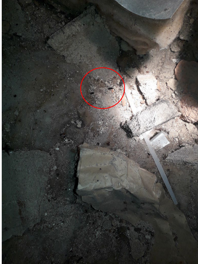
Plate 7. Potential bat droppings near the access hatch of void 1.
