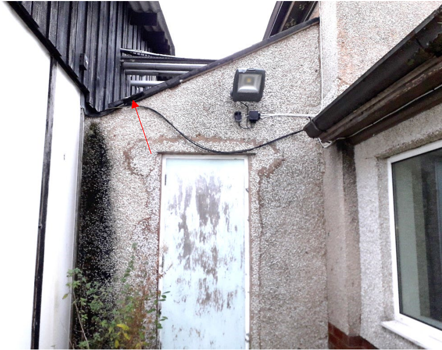
Plate 17. PRF C2 gap in the end tile.
