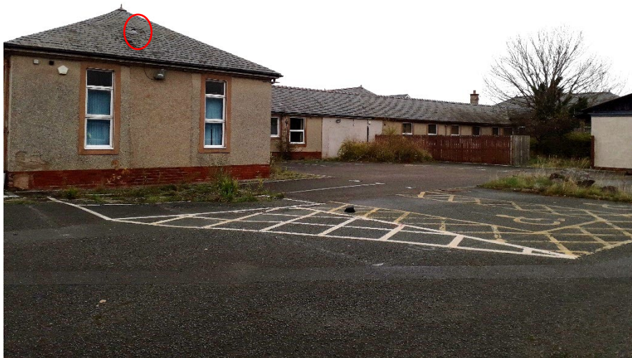
Plate 4. Rear view of the building and PRF A7 – missing slate on hipped end.
