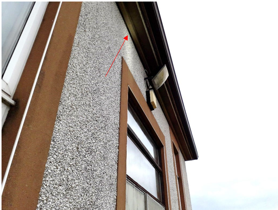
Plate 16. Example of PRF C1 – gap between wall and soffit.
