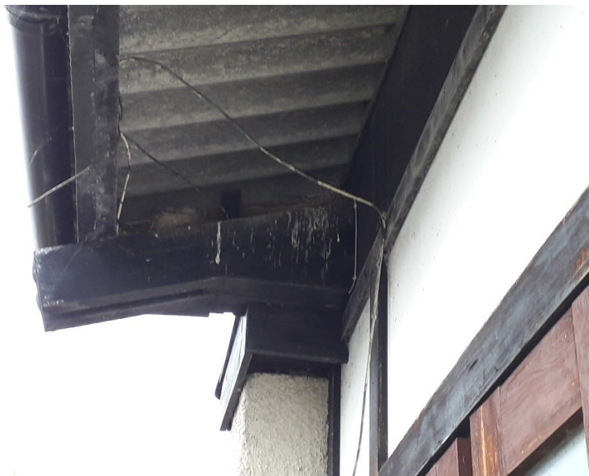
Plate 12. Old birds' nests on the roof frame of overhanging roof.
