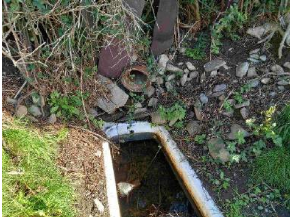
Photograph 13: Bath (TN1) with run off pipe
