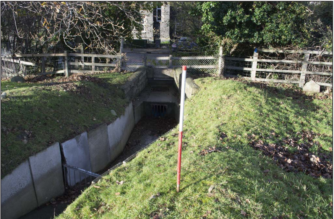
Plate 16: View of modern culvert on the north boundary of the stream with the road; scale 1x1m; view from S (archive reference: G2756_016).
