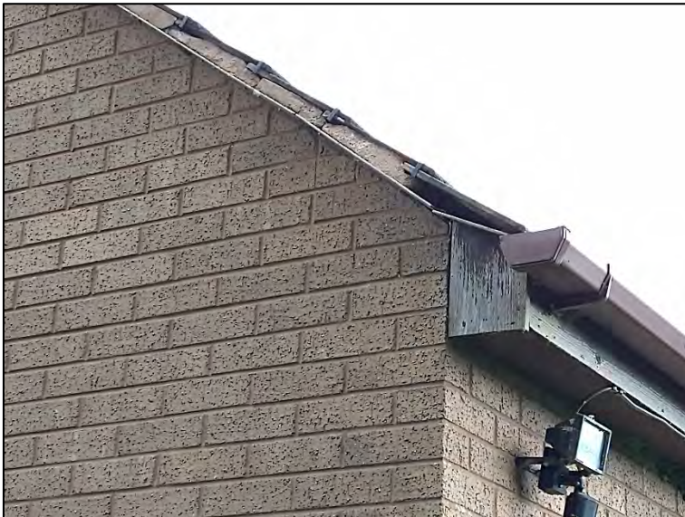
Plate 14: Missing mortar beneath end tiles on summerhouse, potentially allowing access into roof space for bats.
