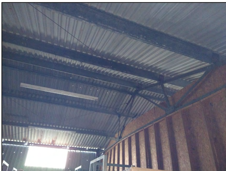
Plate 9: Internal structure of Building 2, showing lack of roof voids and partial chipboard partitioning.
