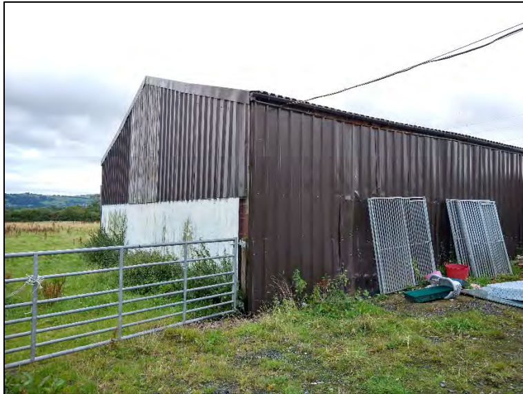
Plate 4: Building 1 (agricultural shed) showing sheet metal walls and roof, with lower sections of breeze block construction.
