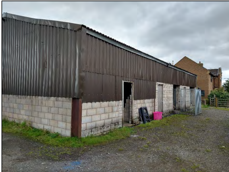
Plate 7: Exterior of Building 2 (agricultural shed) showing breeze block base and sheet metal upper walls and roof.
